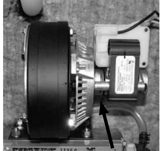
Fan Pressure Switch Hose
