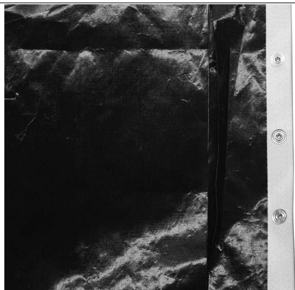
BELT IS TORN AND FOLDED. REPLACE BELT.
