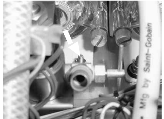
FIG 8 Chilled Water Flow Valve P3487
