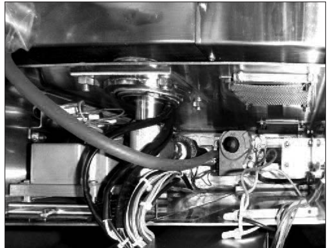
Photo showing manometer hooked up to outlet side of valve.
