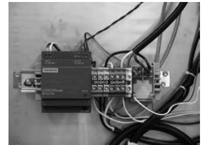
The 24-Volt Power Supply is DIN rail mounted on back of unit.
