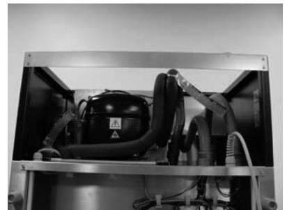
[Photo 2] From rear of unit
