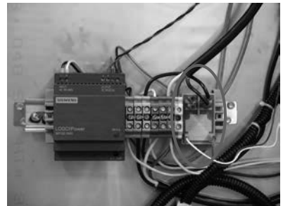
Relay is mounted right of DIN rail-mounted terminal block.
