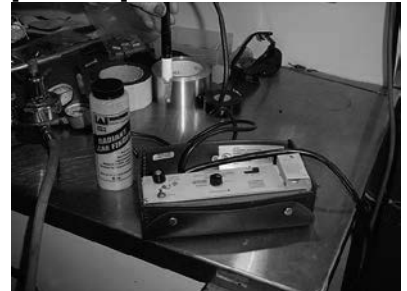
If system pressure is too low or the leaks difficult to pinpoint, pressurize system with 150 PSIG [10.5 Bar] of Nitrogen and use an electronic leak detector or soap solution.
