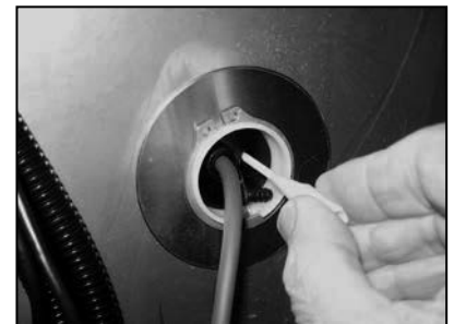
[Photo 2] – From rear of unit
