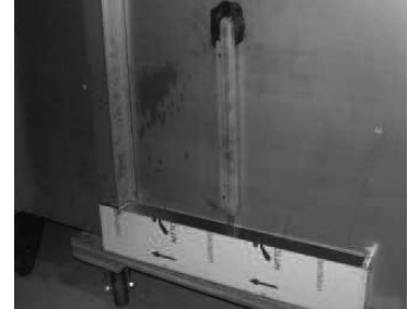
Install rear drain tubing chase to hold elbow at bottom of hole & ensure a drain downward slope.
