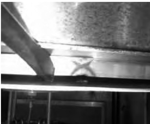
Example of broken weld
