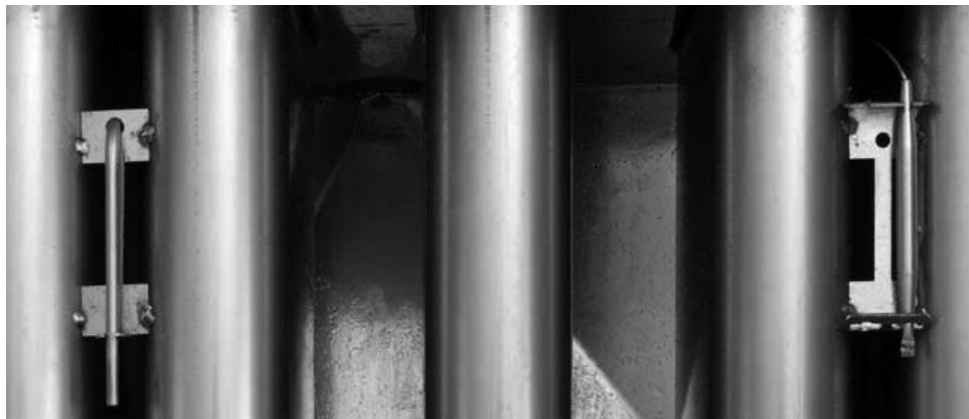
Typical sensor probe/high-limit locations and mounting hardware.
