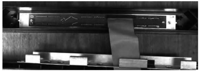
Fig. 8. Note ribbon cable is at top of bezel opening.
