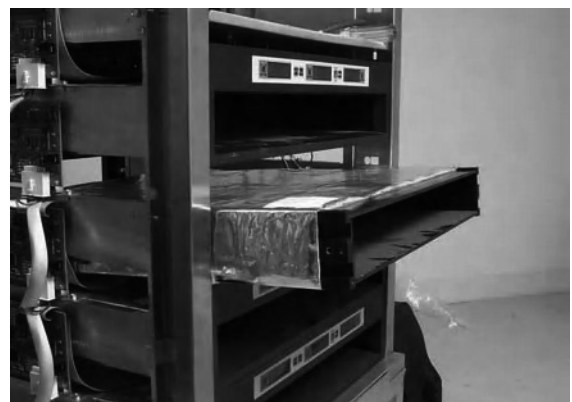
Fig. 17. Slide malfunctioning slot from cabinet.
