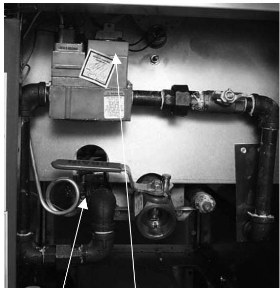
Light pilot here Gas valve
