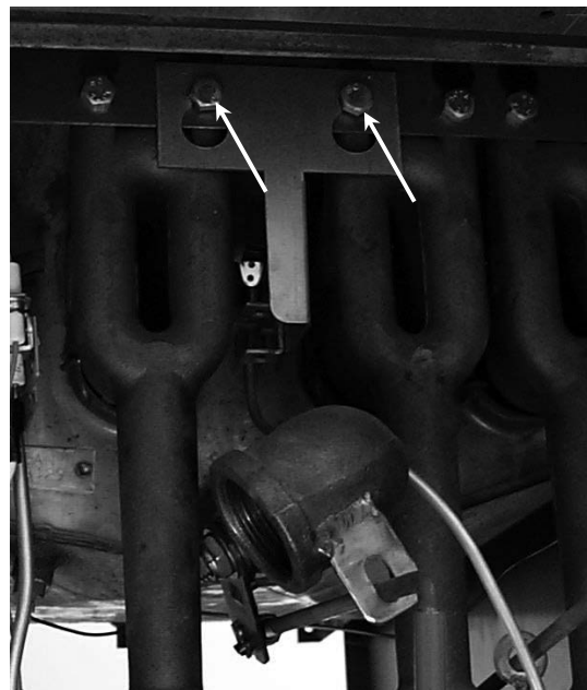
Old-style trailing pilot bracket is mounted on burners.
