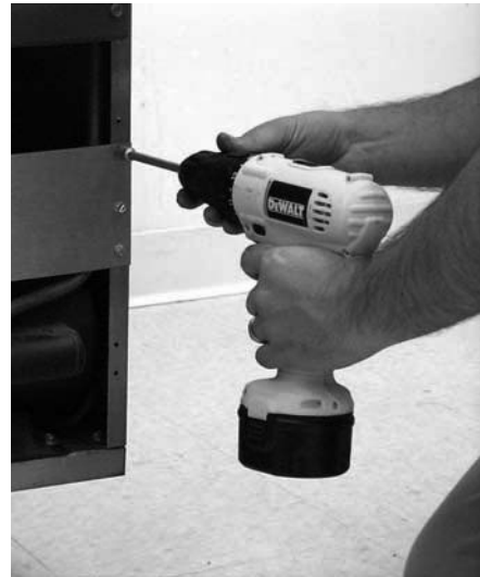
Removing gas manifold shield.
