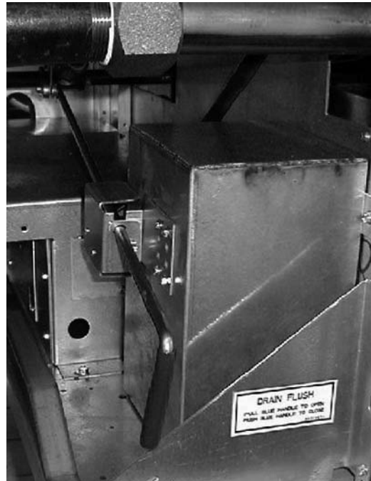
Drain-flush handle (blue) location.
