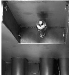
Upper float switch.
