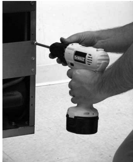
Removing gas manifold shield.
