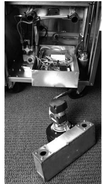
Blower and plenum removed
