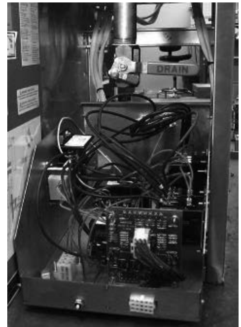
Fig: 10-10 Contactor box partially removed from the
