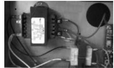
Fig: 10-9 On the surface ship fryer, the transformer is in the controller box.
