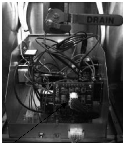
Fig: 10-7 The interface board is in the contactor box in the sub fryer.
