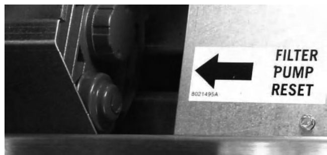
Reset switch location: New-style FPIII
