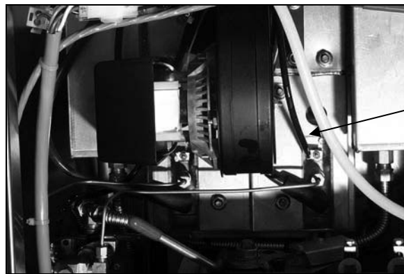
Flame Sensor Wire (Right Burner)
