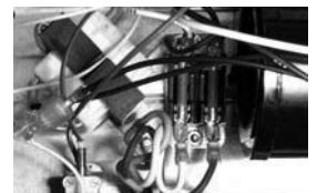
Transformer and fuses.
