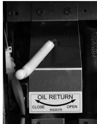
Moving the yellow handle to the open position opens the oil return valve and activates the filter pump.
