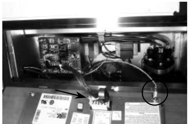
Wire harness/connector and ground wire on controller back.
