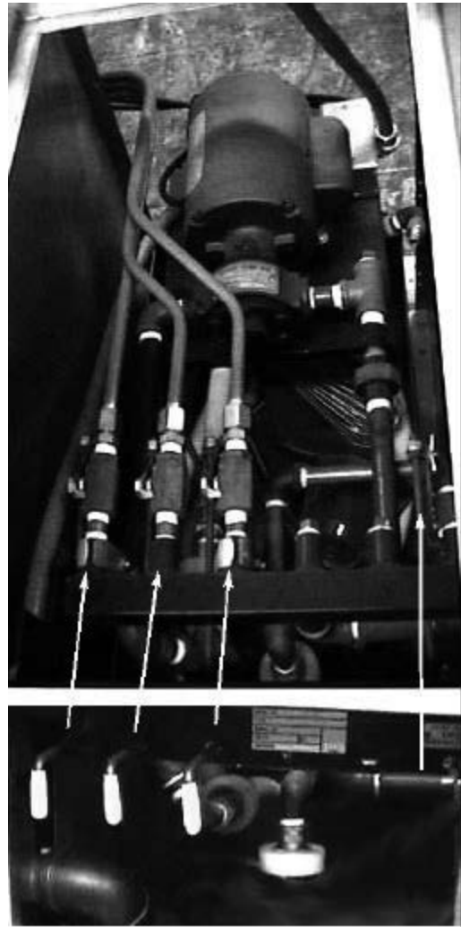
Push-pull variation valve control handles. Yellow handles operate oil return valves, and the red handle operates the hose connect valve.
