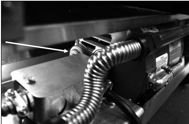
Filter Pump Reset Switch (Arrow)
