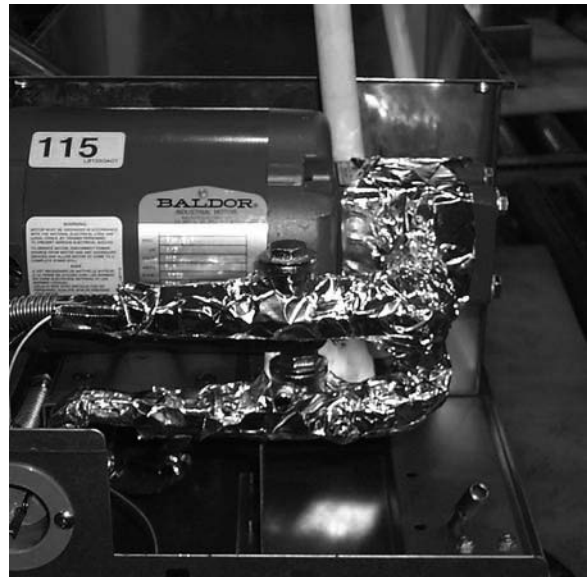
Heater strip installed [115V PF50 (Return/Suction)].
