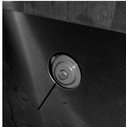
The motor thermal overload switch (arrow) is located on the left side of the filter.
