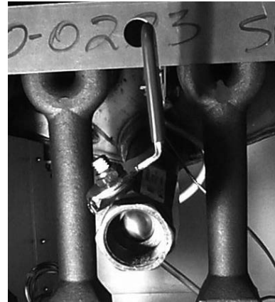
Fry vessel drain valve.
