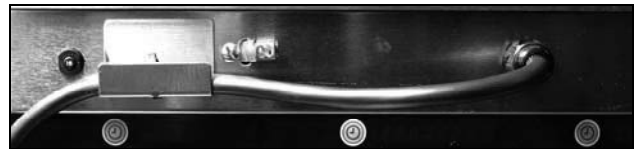
Cord shown resting in hanger. A zip tie holds it in place.
