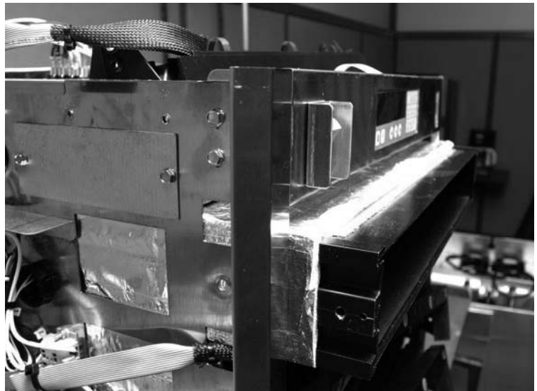
Fig 10: A row is shown partially removed from the cabinet.
