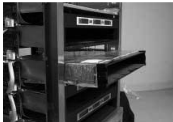
Fig. 17. Slide malfunctioning slot from cabinet.
