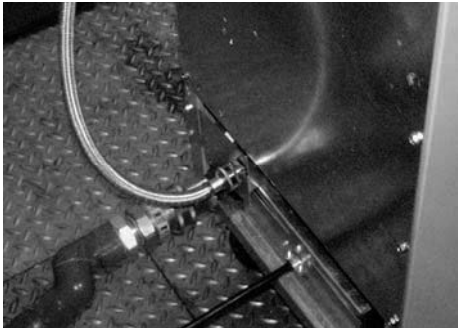
Gas. Water Connections
