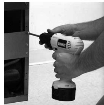
Removing gas manifold shield.
