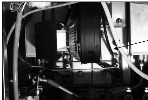
Flame Sensor Wire (Right Burner)
