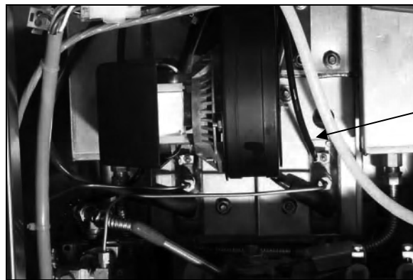
Flame Sensor Wire (Right Burner)
