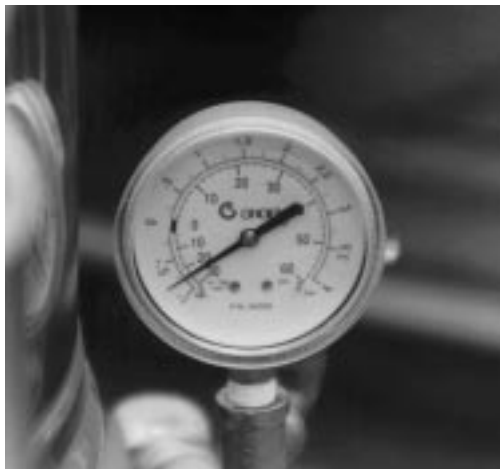
The pressure gauge should show a vacuum of 20 to 30 inches when the kettle is cold.
