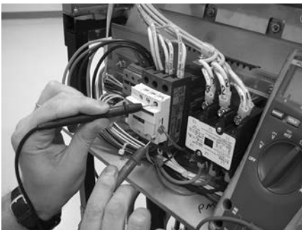
Heat contactor ohm check
