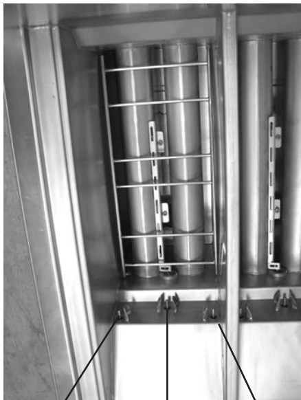
Oil level probe Temperature probe Oil level probe
