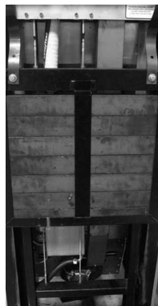
View of the counter-weights with cover removed
