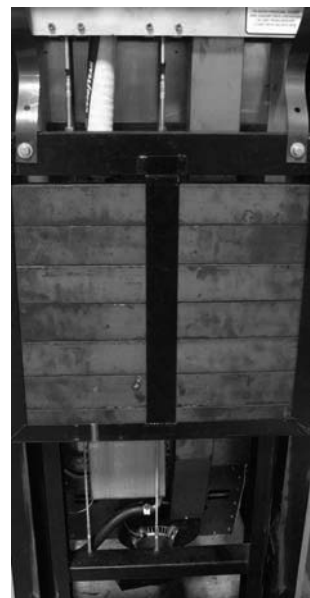
View of the counter-weights with cover removed
