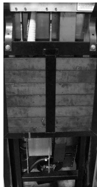
View of the counter-weights with cover removed
