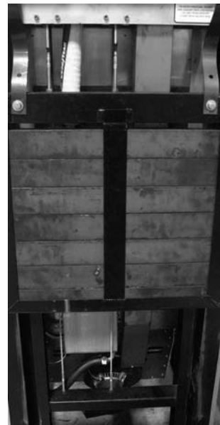
View of the counter-weights with cover removed
