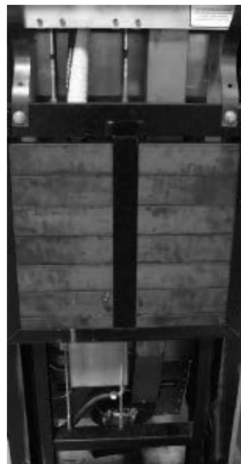
View of the counter-weights with cover removed
