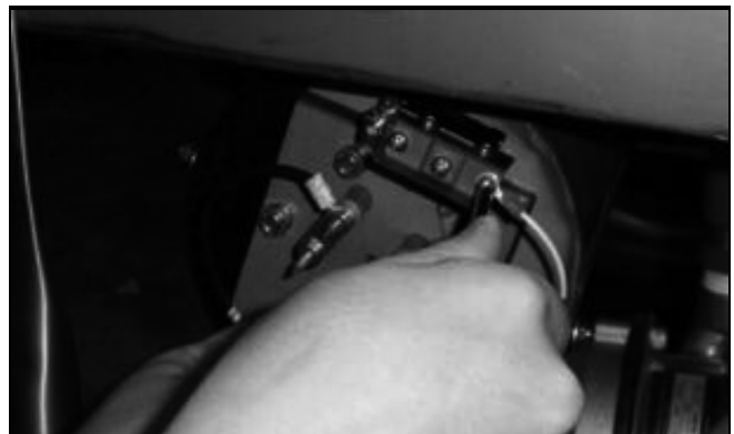
Securing jumpers to the thermostat.
