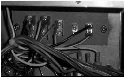
Terminal board inside the heater box
