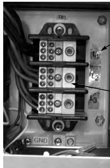
Incoming Power Connection
