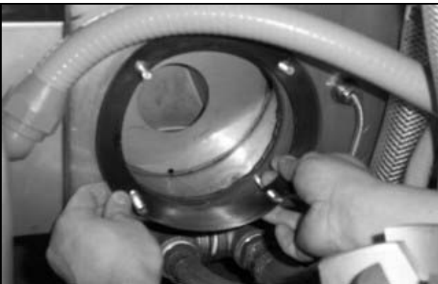
Removing the pump gasket
