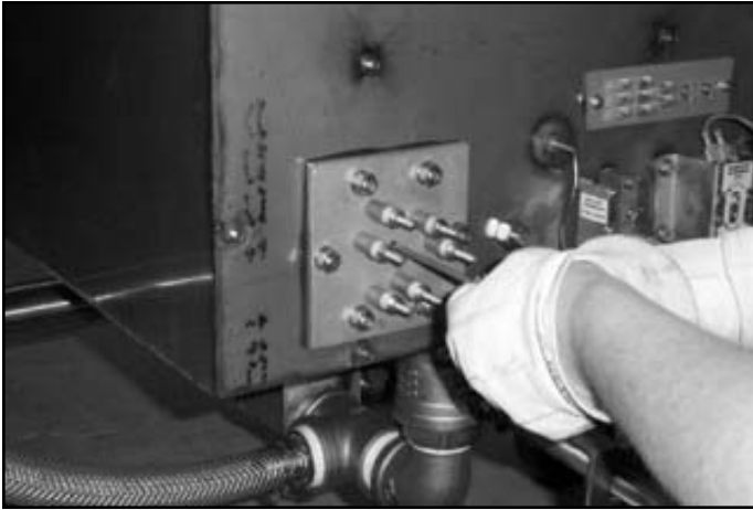
Putting the thermostat probe in the heater well
