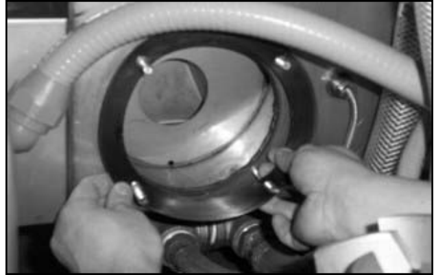
Removing the pump gasket
