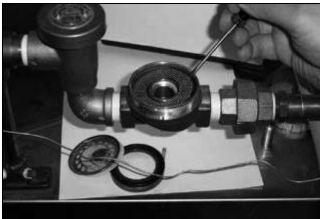
Removing the mesh strainer screen
