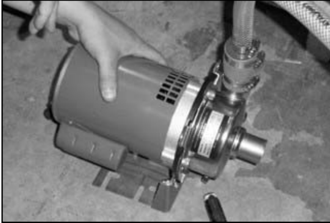
The assembly removed from the unit.
