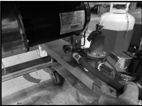
C. PRV Inlet from Coil
