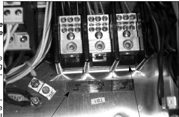
Incoming Power Connection
