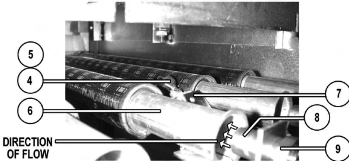
Gas Train, 200K Boiler Shown
